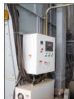
稻壳炉控制系统 STOVE ELECTRICITY CONTROL SYSTEM
